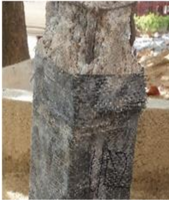
Figure 4: Typical Failure mode of the CFRP Wrapped Specimen
